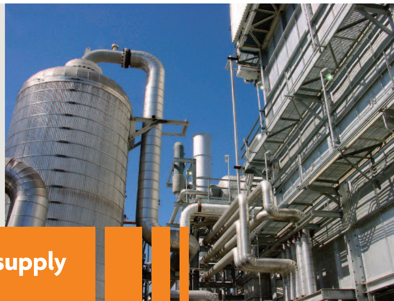
USA - 31,000 Nm 3 /h Hydrogen
