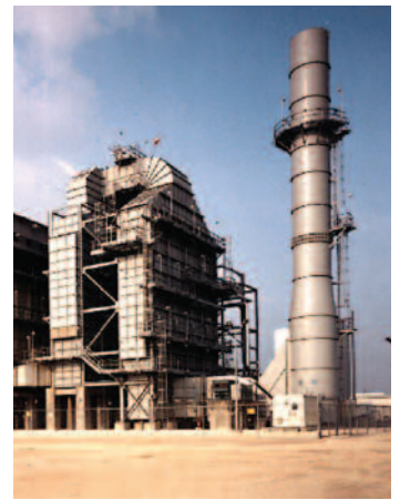
USA - 105,000 Nm 3 /h Hydrogen
