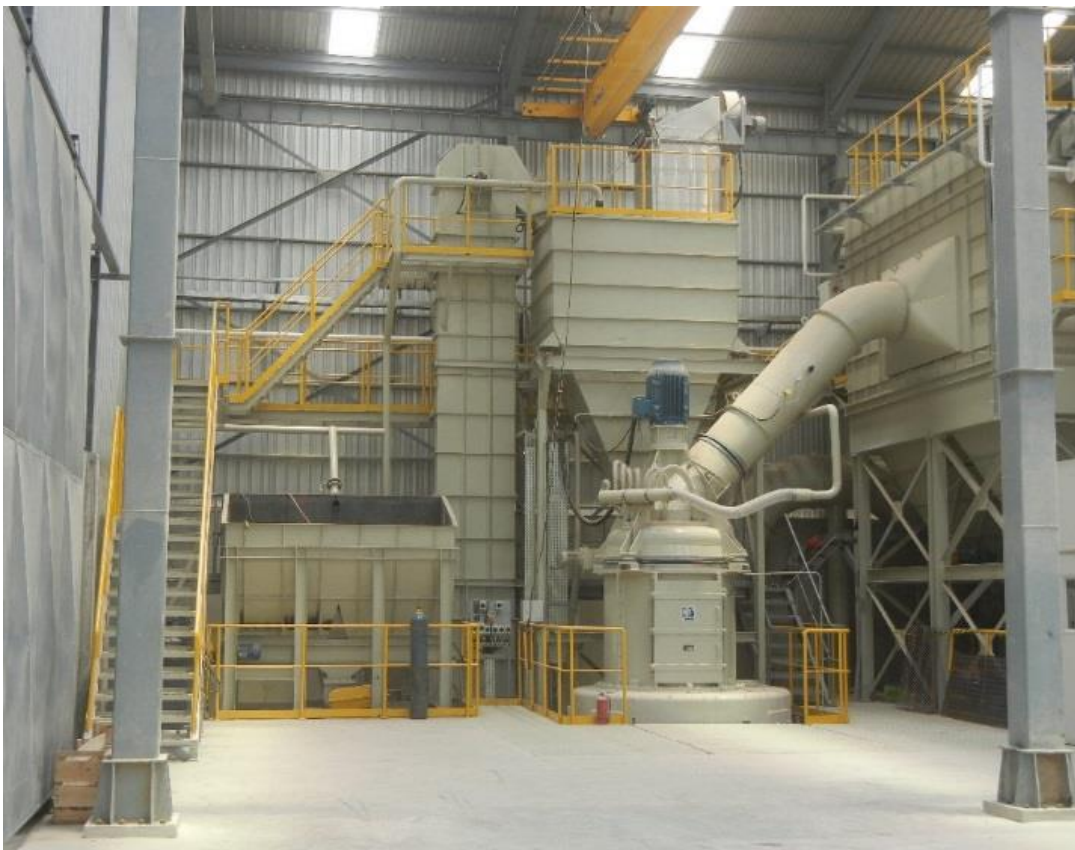
Clariant's new bleaching earth production site increases the regional production capacity for bleaching earth by 35%. (Photo: Clariant)
